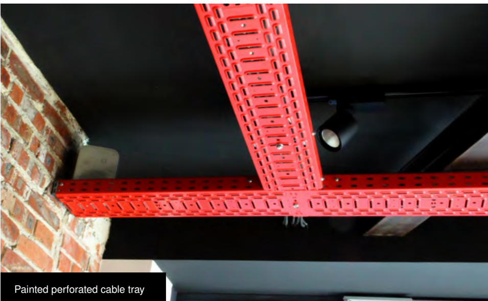
Painted unperforated cable tray Brezel Museum, Erdmannhausen
